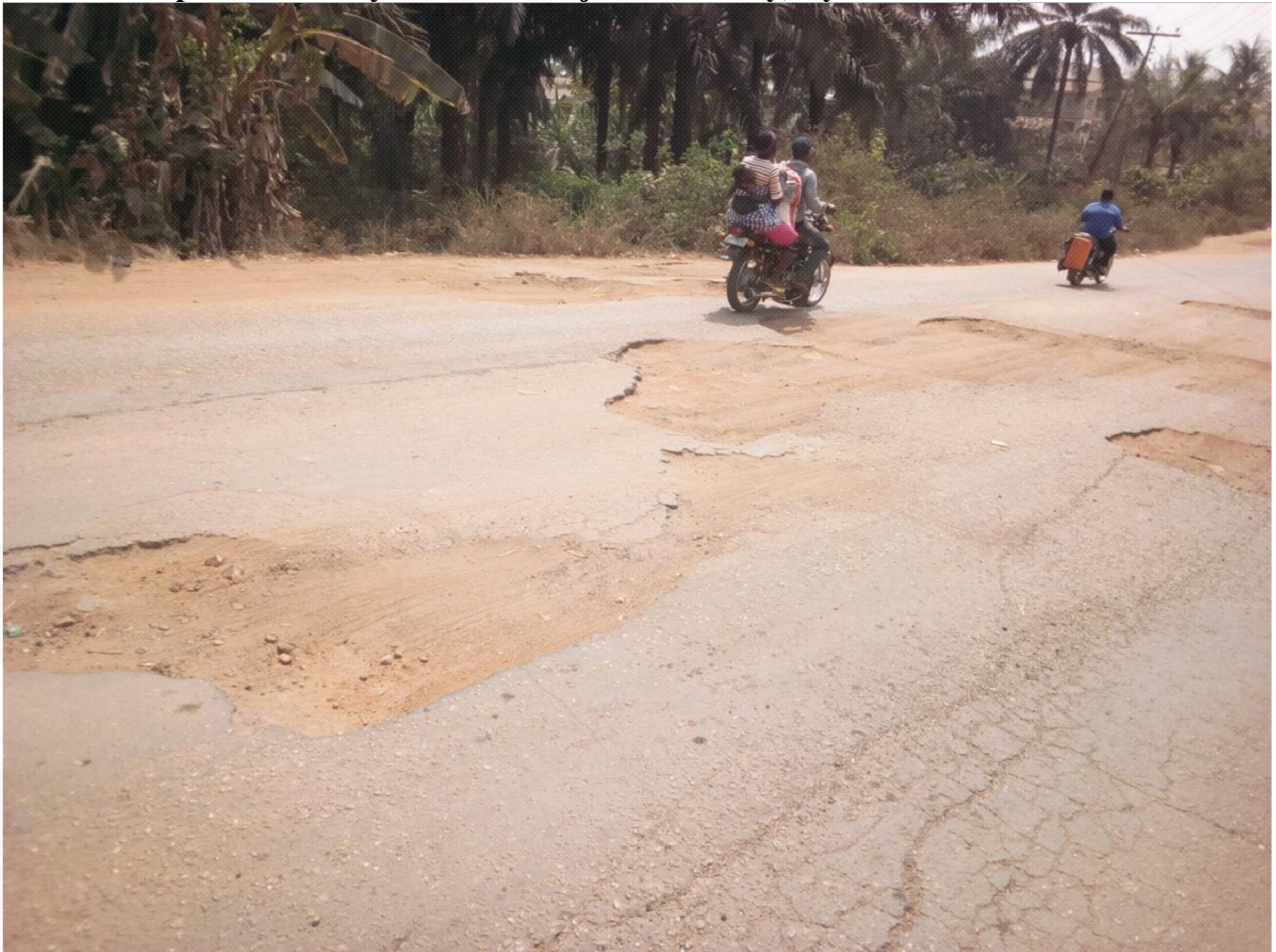
Plate 6: Condition of roads at Oke-Bola Community, Ayedaade LGA, Osun state
