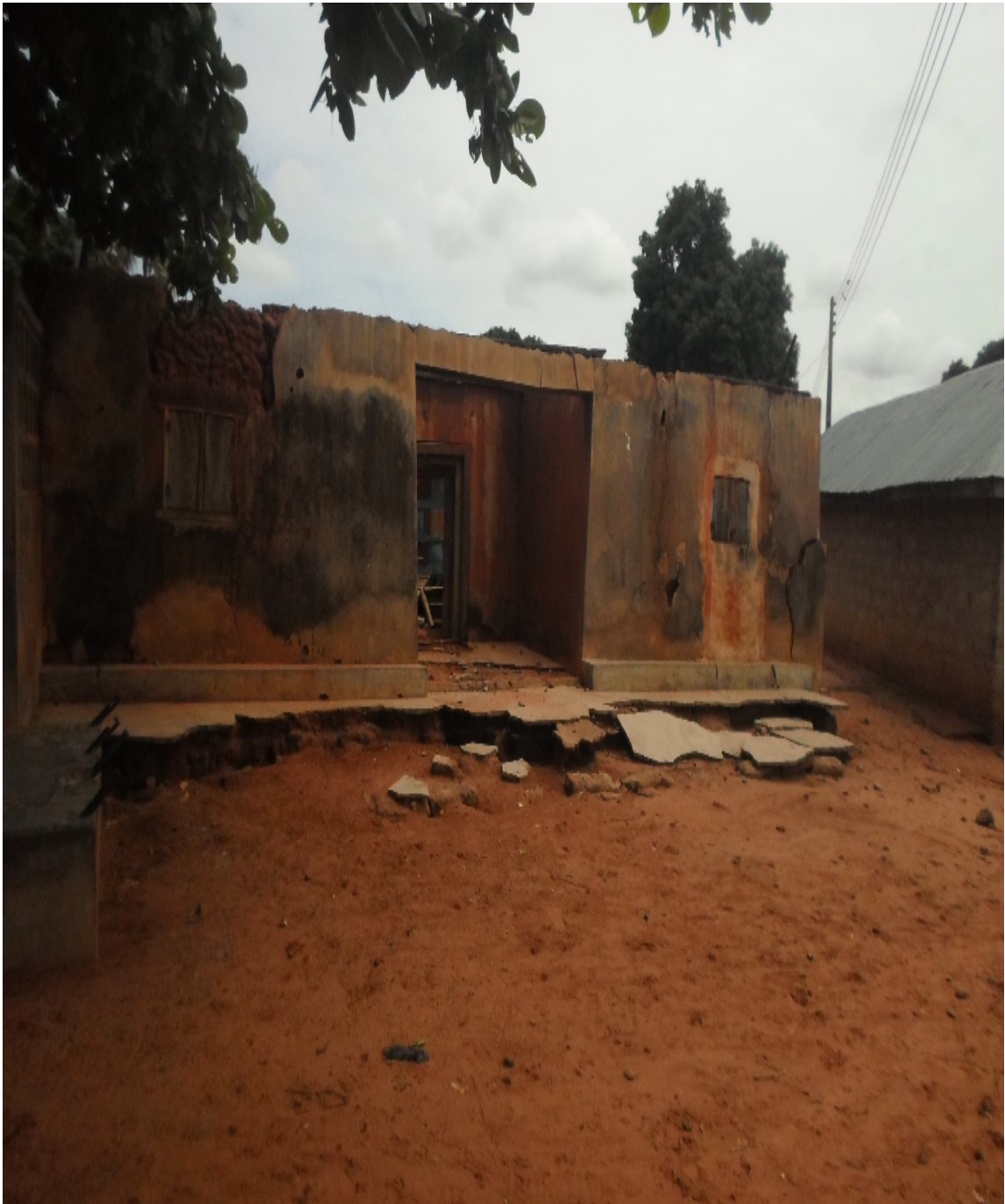
Fig. 5: Collapsed TBS clinic accommodation built by the LGA at Patidzuru, Edu LGA of Kwara state
