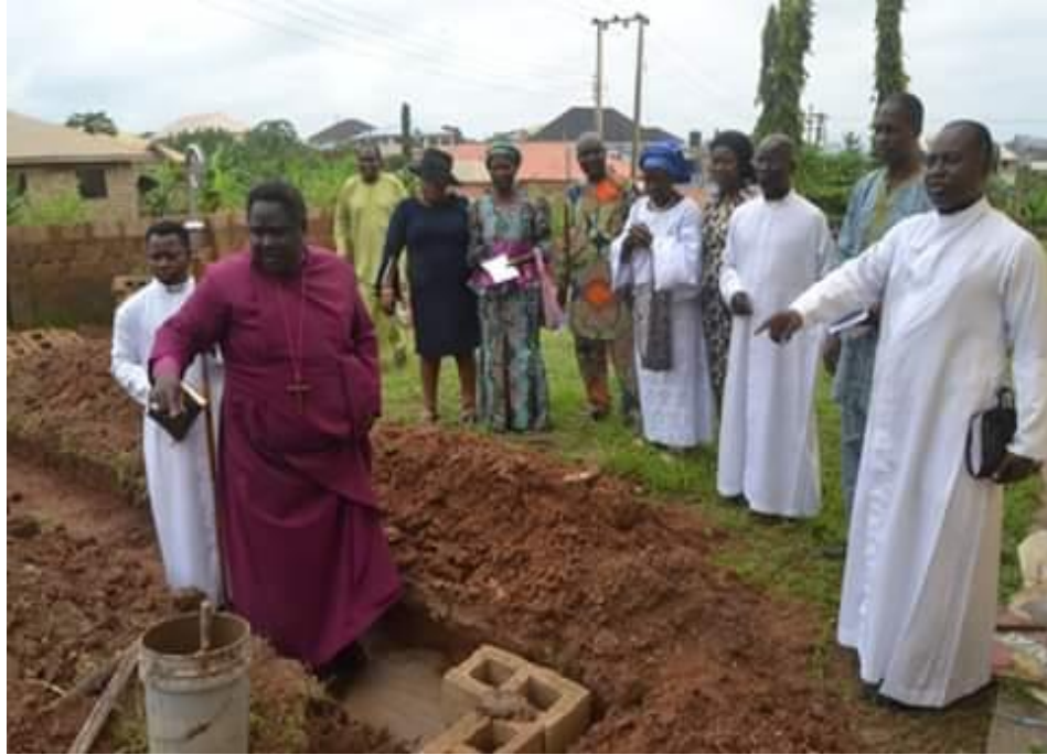
Plate 9: LAYING OF FOUNDATION OF A NEWLY ESTABLISHED CHURCH UNDER IBADAN MAIN DIOCESE LED BY THE BISHOP OF IBADAN DOICесе, HIS GRACE, MOST REV'D (DR.) J.O. AKINFENWA (STRATEGY FOR CHURCH GROWTH AND EXPANSION)
