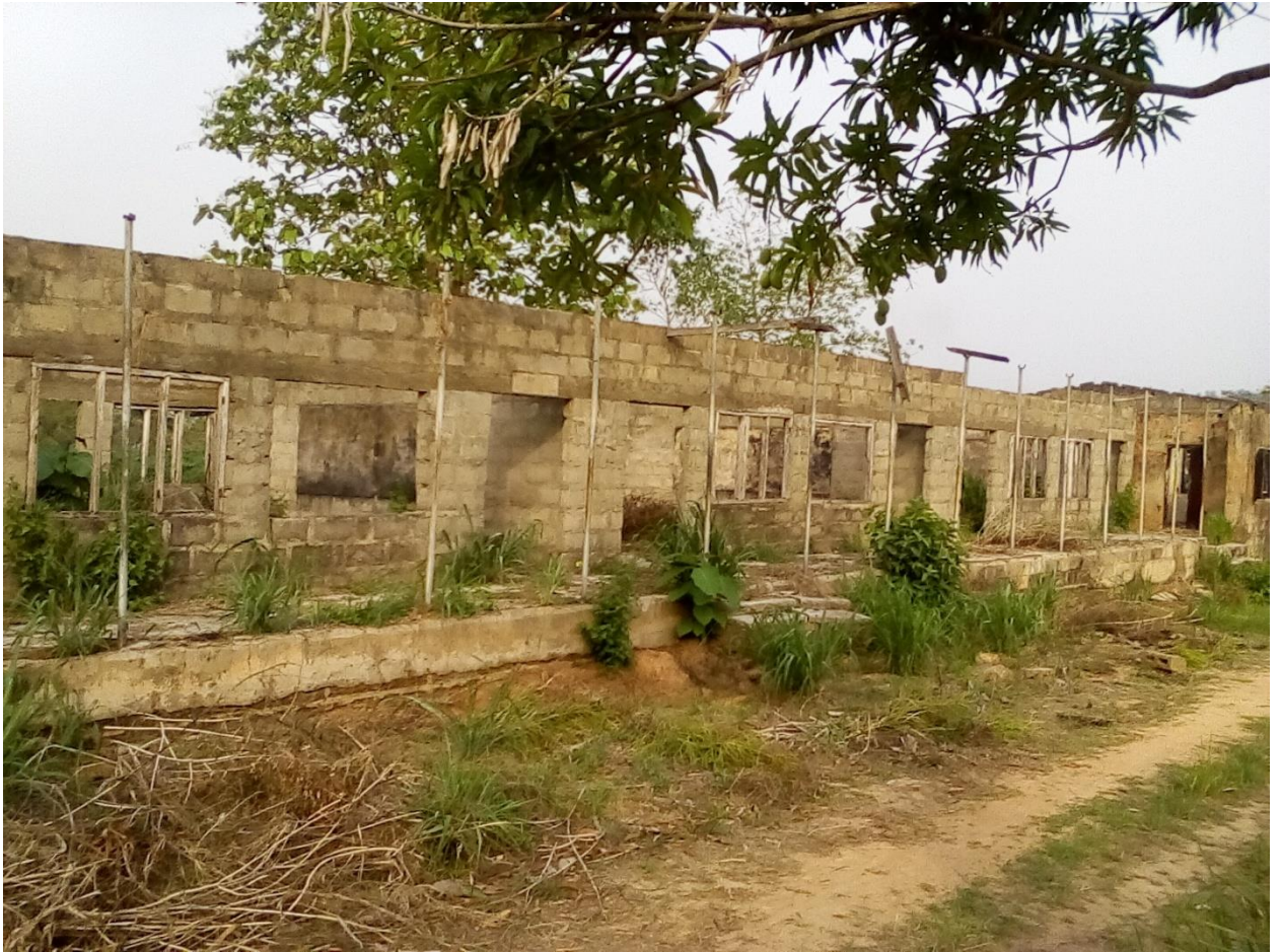
Plate 4.1: Adadama Community Secondary School destroyed during the 2015 boundary conflict
