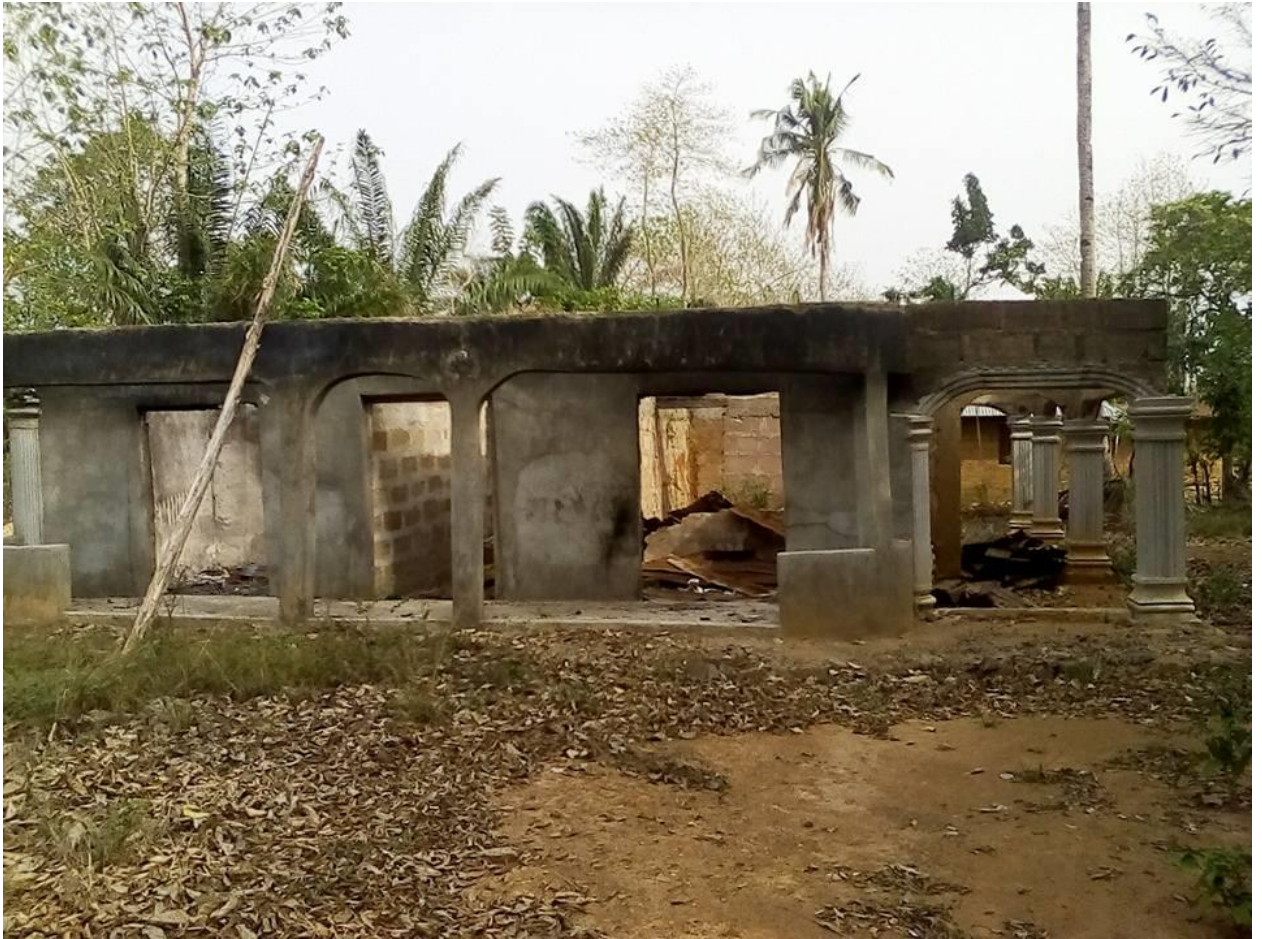
Plate 10: Residential building destroyed in Amagu community during the 2014 conflict
