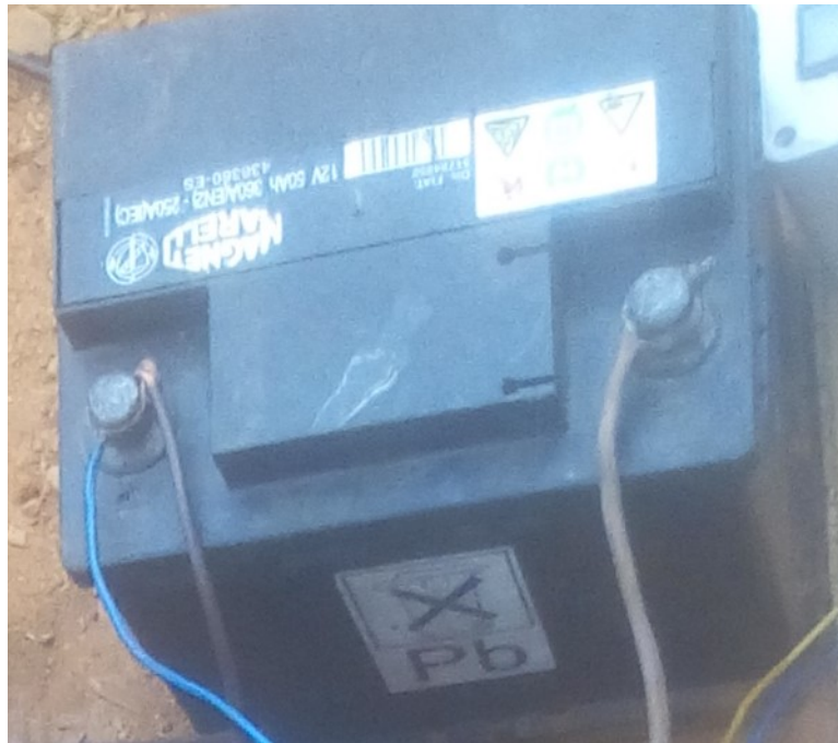
Plate 3.7: 12 Volts DC Battery
