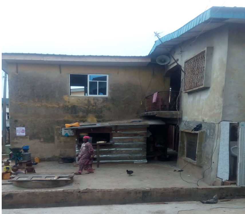
Plate12: A residential building containing a Mosque with loudspeaker mounted on it at Orogun, Ibadan.
